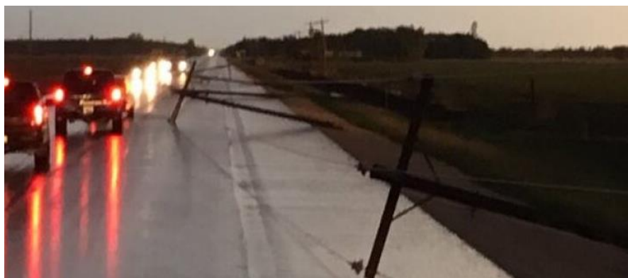
Poles knocked down along Highway 8. By Manitoba Hydro on Twitter
