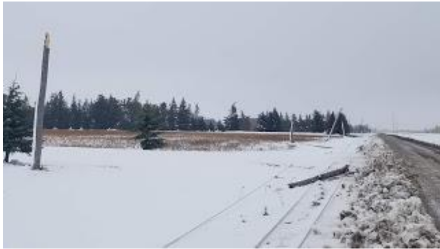
Snapped power poles near Portage la Prairie. By Kyle Brittain for The Weather Network
