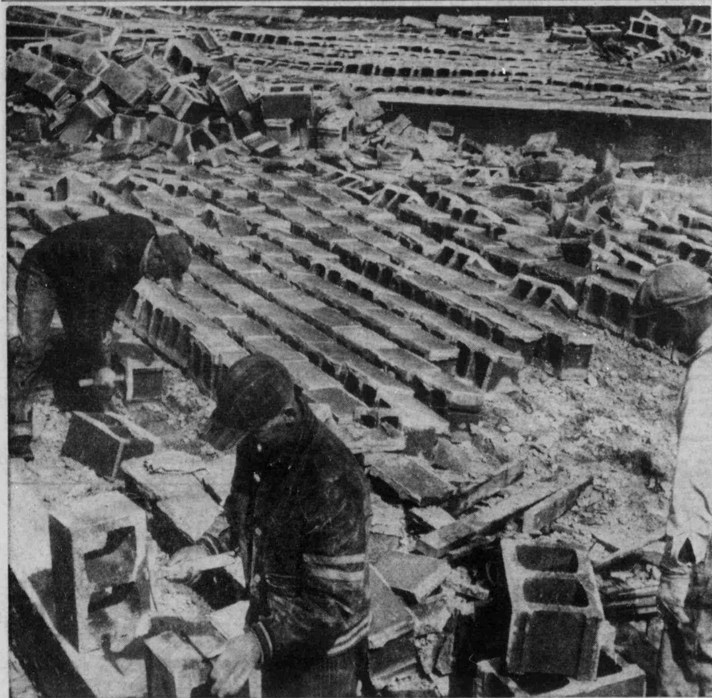
THE WIND DID IT: Masons are busy repairing the damage to this concrete block building which blew down some time last night from 68-mile-an-hour winds. One wall collapsed inward and the other outward at Bannatyne Ave. —Photo by Gordon Aikman.
